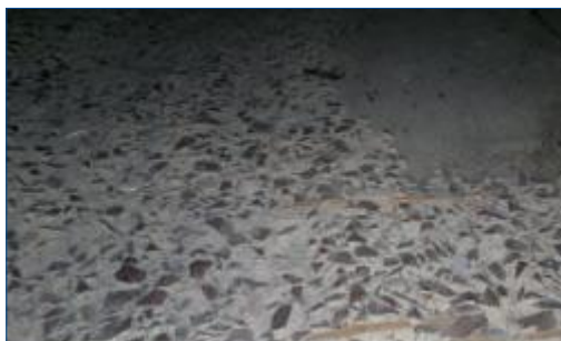
Worn reinforced concrete channel
