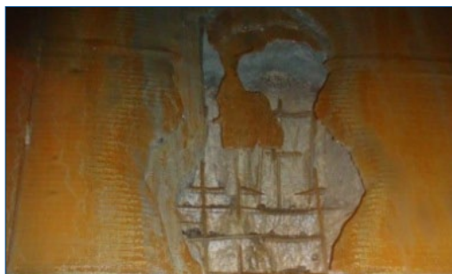
Damaged areas of the concrete sump
