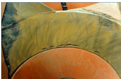
Failed rubber lining
