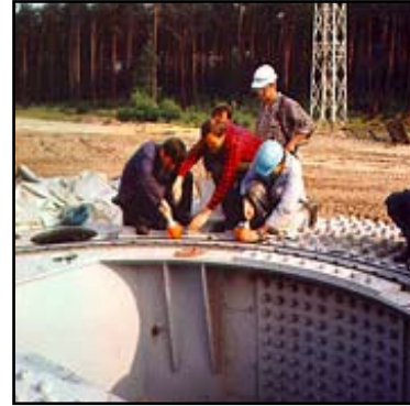
A team of applicators was required to apply all the Belzona® 1111 quickly, to allow time for the rings to be located
