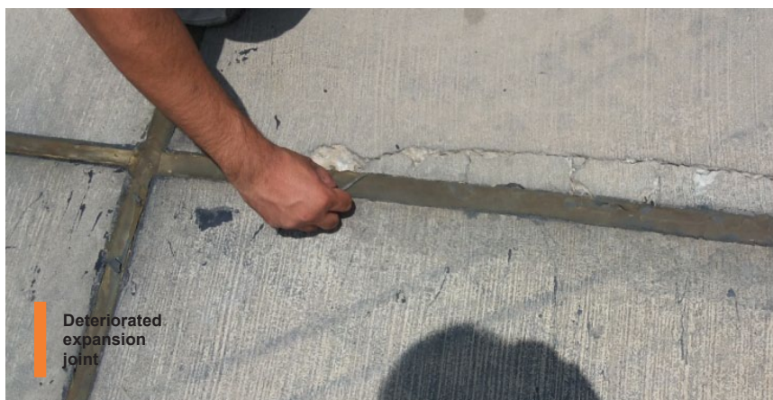
Cracked and spalled concrete
