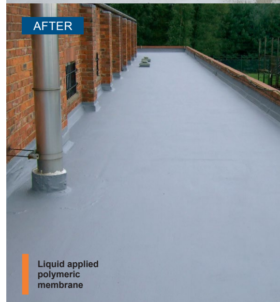
Leaking asphalt roof
