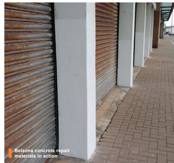
A series of concrete pillars required repair
