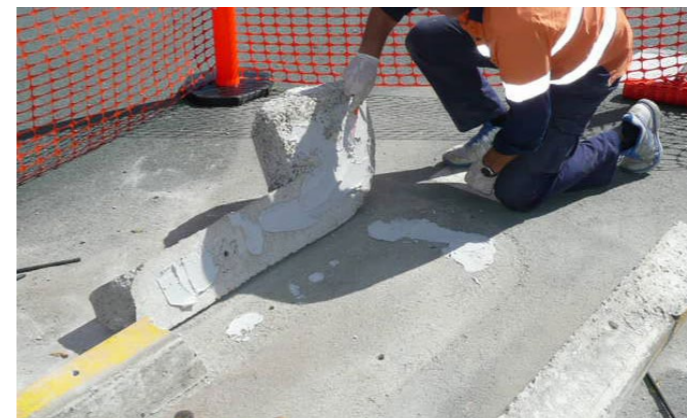
p.20-21 Tackling car park troubles at Australian shopping centre
