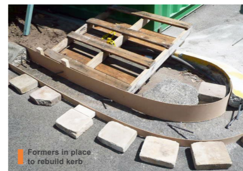
Damaged and disbonded kerb
