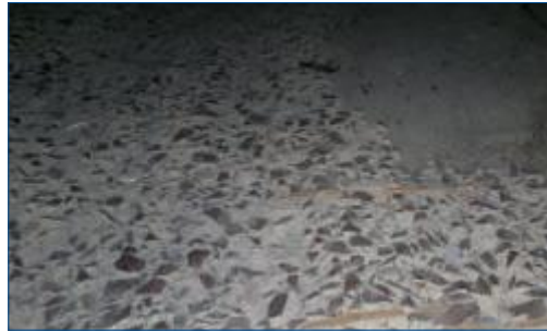
Worn reinforced concrete channel
