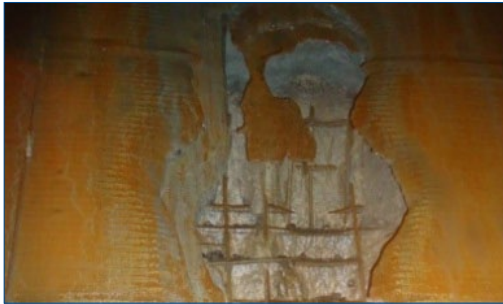
Damaged areas of the concrete sump
