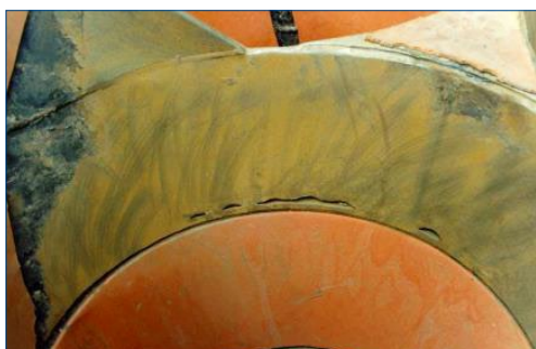
Failed rubber lining
