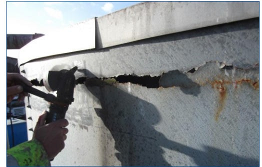
Close up of corroded areas
