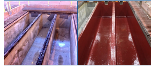
Furniture rails at copper mine protected from CuSO 4 electrolyte
