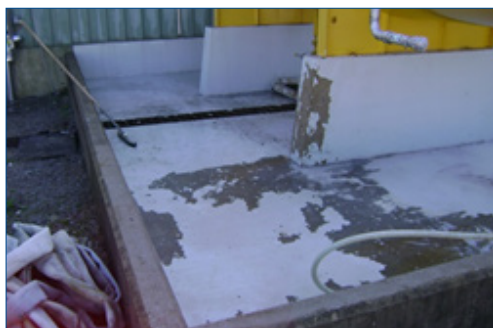
98% sulphuric bund in need of repair
