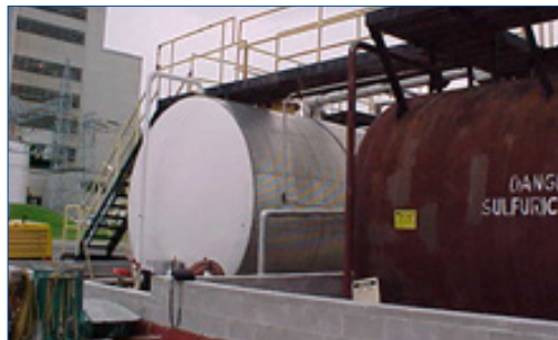
Sulphuric acid (right) and caustic (left) containment areas
