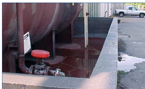
Concrete damage due to system failure
