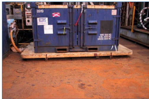
Corroded platform deck
