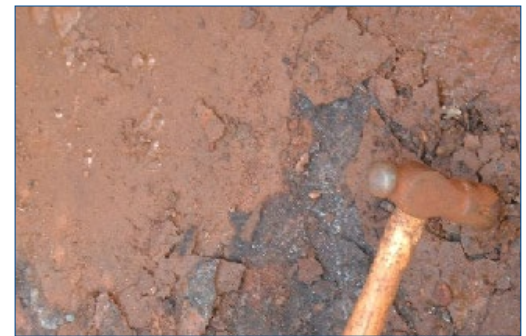
Close up: corroded platform deck
