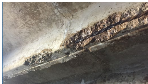
Deteriorated overhead concrete on car park
