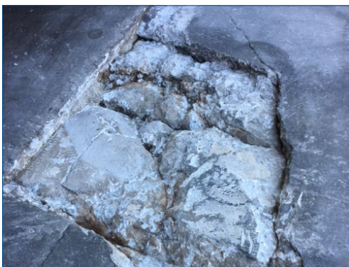
Impact from heavy traffic can damage concrete
