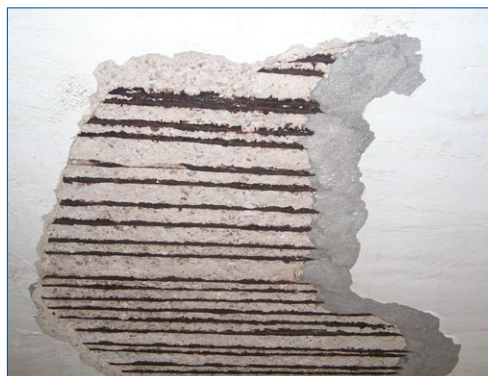
Corroding metal leads to spalled concrete
