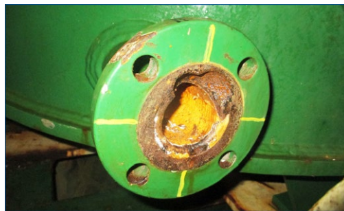
Flange face highly corroded
