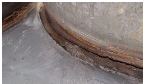
Deteriorated joint on HVAC unit
