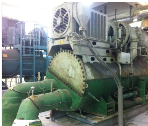
The York chiller unit
