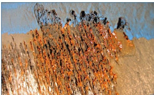
Fig 1: Cavitation damage on a stay vane
