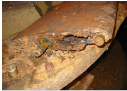
Damaged wicket gate blade
