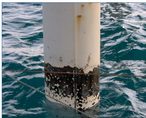
Corroded platform leg
