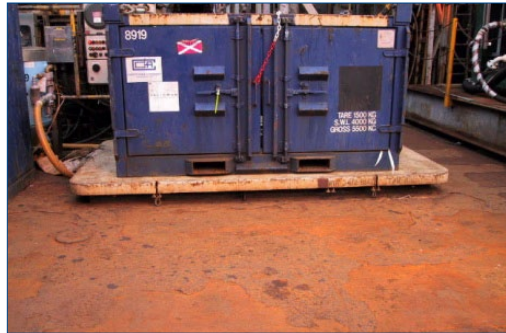
Corroded platform deck
