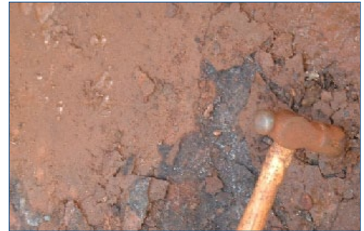
Close up: corroded platform deck
