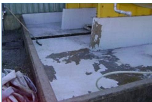
98% sulphuric bund in need of repair
