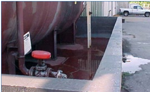
Concrete damage due to system failure
