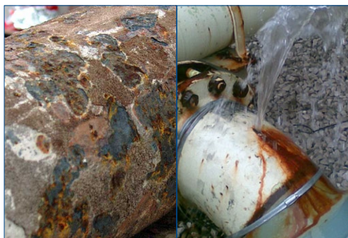
Fig 1: Erosion, corrosion and pitting damage Through wall damage resulting in leaks
