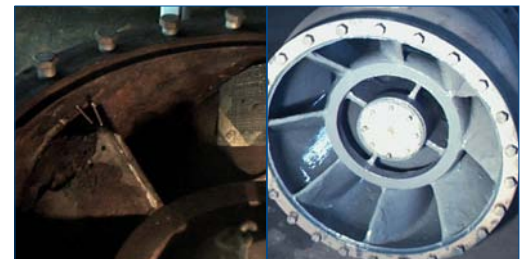
Diffuser vanes with steel gauze in place Completed application
