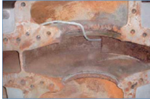
Corroded and cavitated pump
