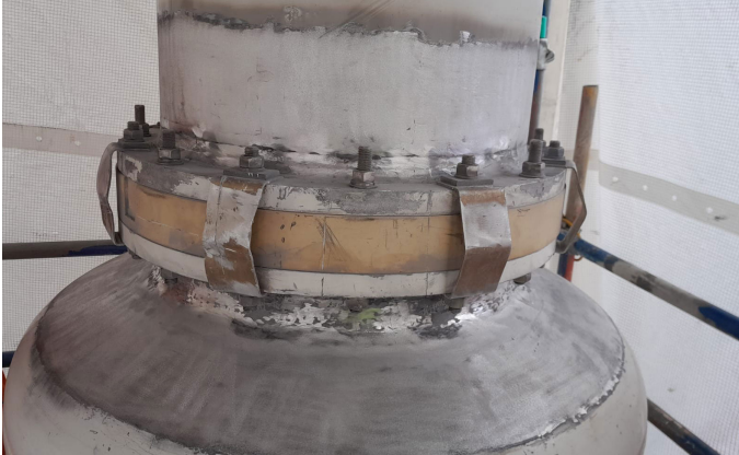
Flange leaking SF 6 gas
